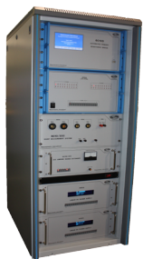
Figure 1— 6010/300 A System with Front Connections
